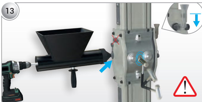
After the initial filling, tap the busbar block joint from underneath with a plastic mallet. If a drop in the Flex-Comp level is observed in the level control plastic, continue the filling process.
